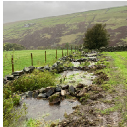
Natural Flood Management Works completed under Calderdale Metropolitan Borough Council funding (CCRT)
